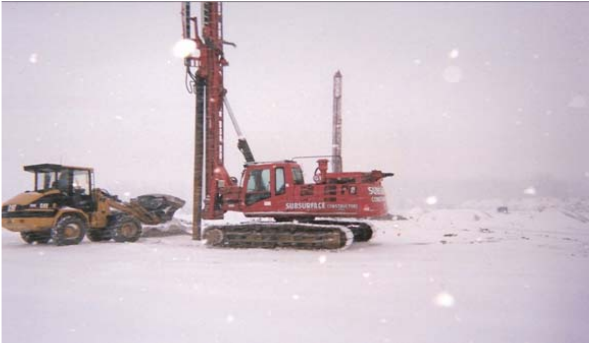
Bluffton, IN Bio Energy Ethanol Plant – Vibro Stone Columns for Tank Foundations
