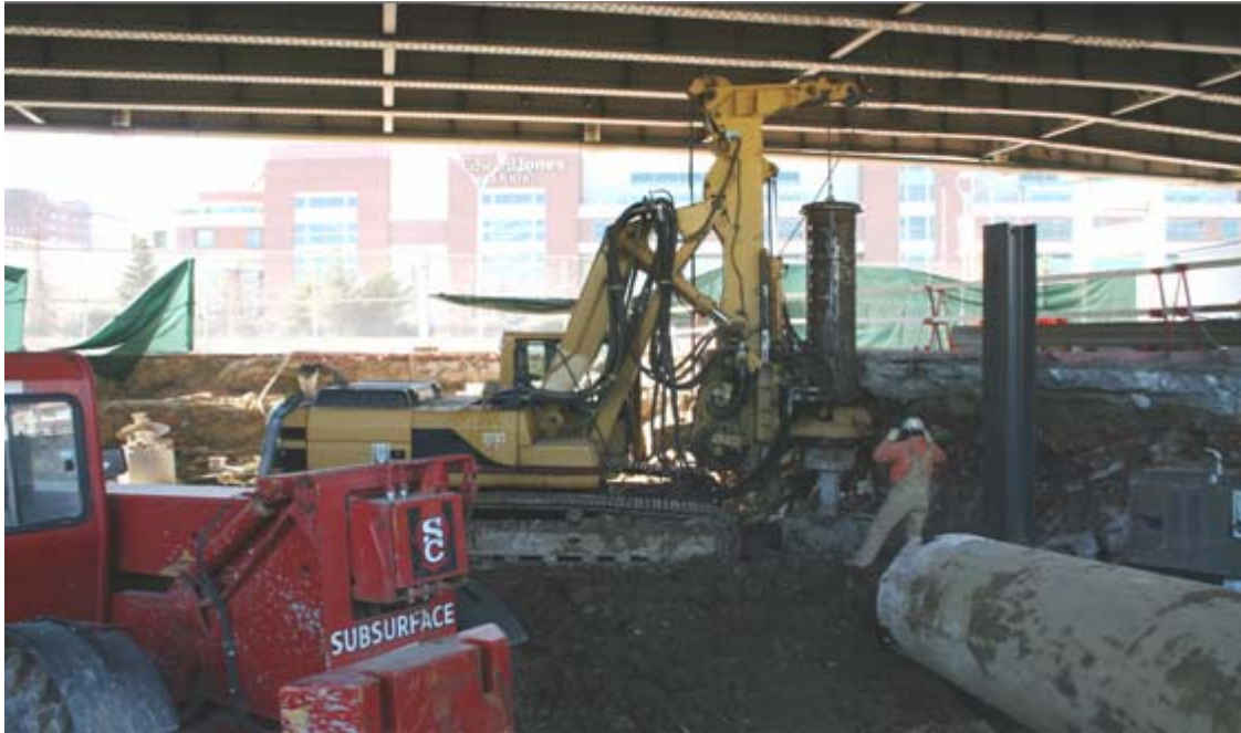
Pinnacle Casino Tunnel, St. Louis, MO – Earth Retention for Cut and Cover Tunnel
