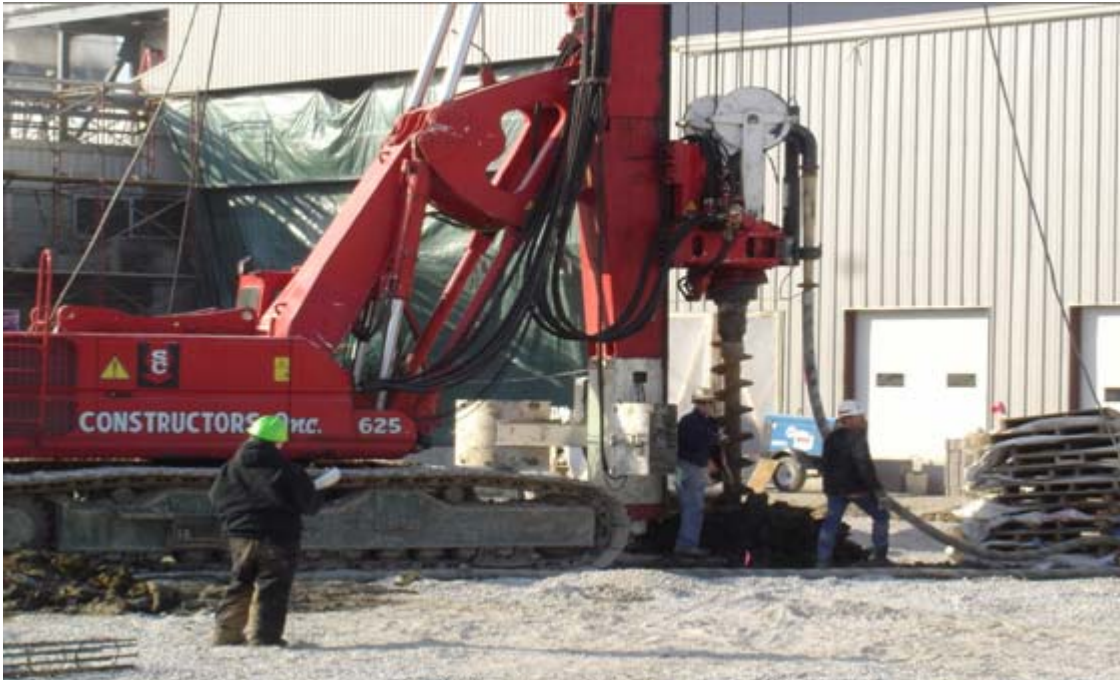
Proctor and Gamble PCC Building – Iowa City, IA – Augercast Piles for Building Addition
